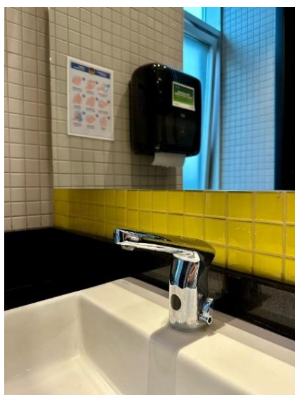
Image 7. Faucet Systems with Aerators
