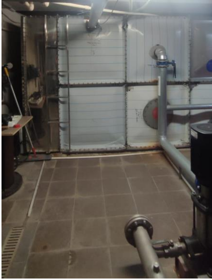
Image 3. Plumbing Infrastructure for Wastewater
